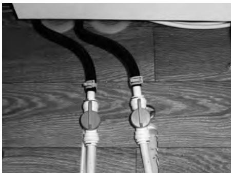
Ventile in offener Position
